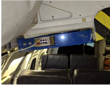
Figure 1: Network Switch Box
