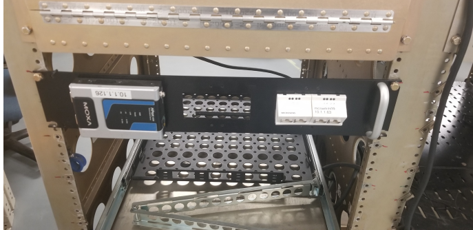
Figure 3: Rack Mountable Switch and RS-232 Converter
