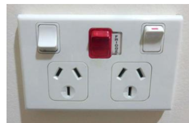
Typical outlet in Fiji
