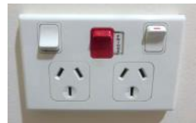
Typical outlet in Fiji
